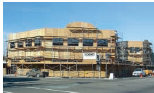
This 20,000 square foot commercial building at 401 Healdsburg Ave. in Healdsburg will be part of the already bustling downtown area. GCCI is the general contractor.
