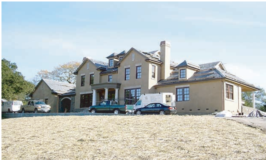
Total Concepts is currently building this custom home in Shiloh Estates with a building schedule of 14 months from start to finish.
