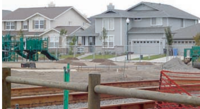
Windsor's Vintage Greens community has a 4-acre park under construction with play structures in place. Homes in the background are occupied.
