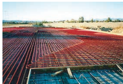
Sonoma-Cutrer's Grand Cru Cellar ceiling with radiant cooling pipes before the 8-inch concrete topping slab was poured.
